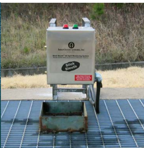
Figure 7. Unit deployed over deep sump at a GenCo in the US. Automated control of sump pump discharge. Photo courtesy Entergy.
