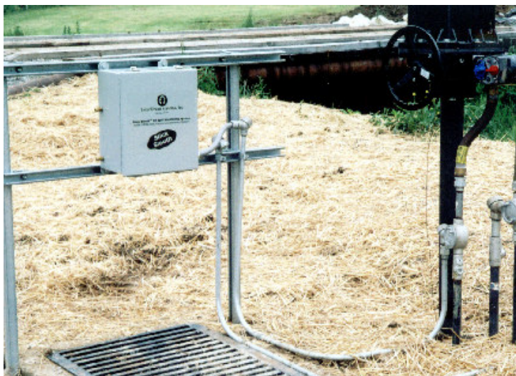
Figure 5. Oil detector operating over stormwater sump. Real time output to nearby control center, and automated shutoff of sump pump.
