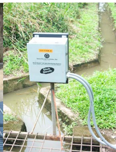
Figure 8. Discharge monitor installed at production facility in Ecuador. Photo courtesy Occidental.
