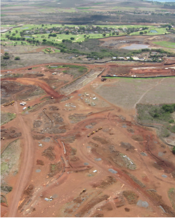
Land clearing for coastal development leads to increased sedimentation on coral reefs delivered in stormwater runoff. Source: NOAA (credit: J. Kozłowski)
