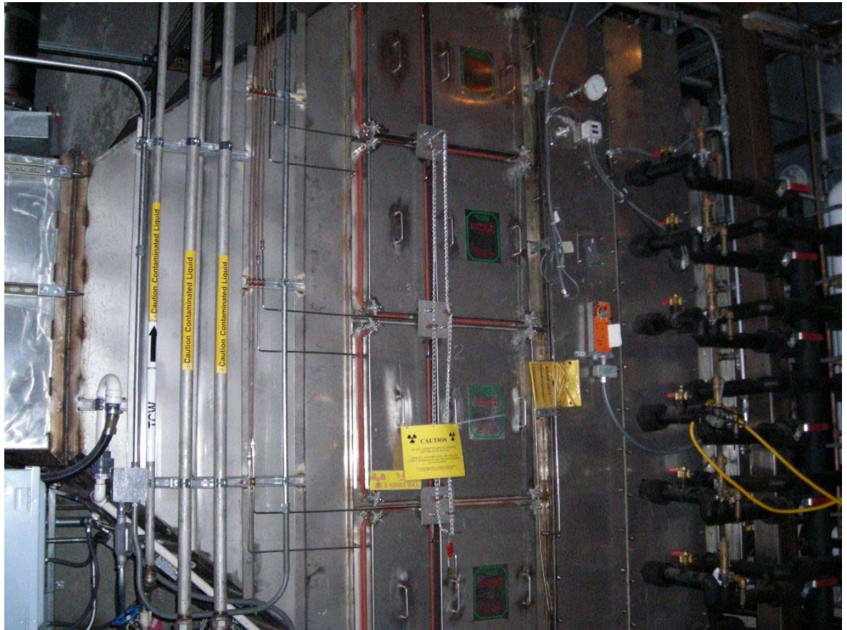
NuMI Target Chase Ventilation Bank
