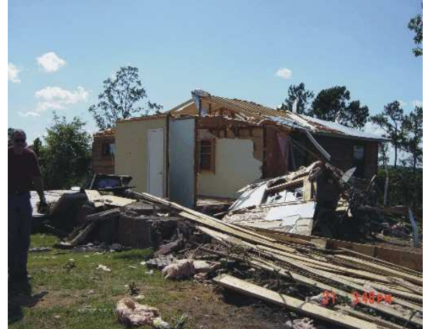
A house in Walnut, MS is severely damaged by a F1 tornado during Memorial Day Weekend. Photos by Scott Cordero
