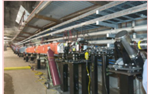
Under construction: the NuMI beam line (Click on image for larger version.)
