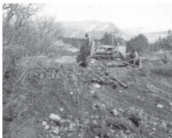
Figure 11 —Pipe harrow and Hansen seed dribbler being used to seed shrubs and cover herb seeds to improve interspaces between pinyon and juniper trees and Gambel oak. Herbs were broadcast seeded prior to treatment.
