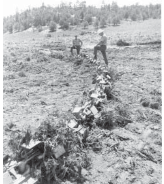
Figure 7—Dixie Sager. Anchor chain with railroad rails welded horizontally to both sides of each link.
