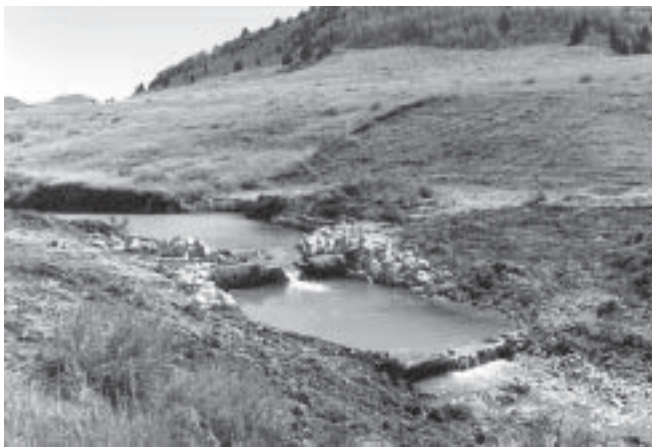
Figure 8 —Channel reshaping and construction of impoundments may be required to stabilize stream channels prior to seeding and planting.
