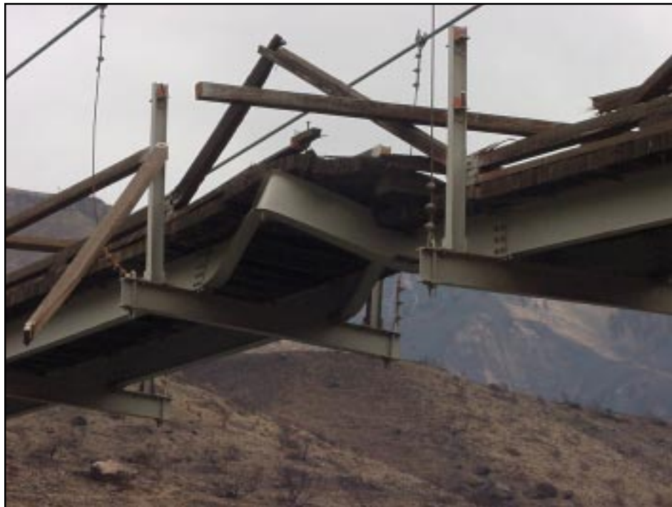
Bernard Bridge buckling from fire damage.
