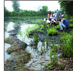
Students help install soil-bioengineering practices to improve coastal marsh habitat on Grosse Ile, Michigan.
