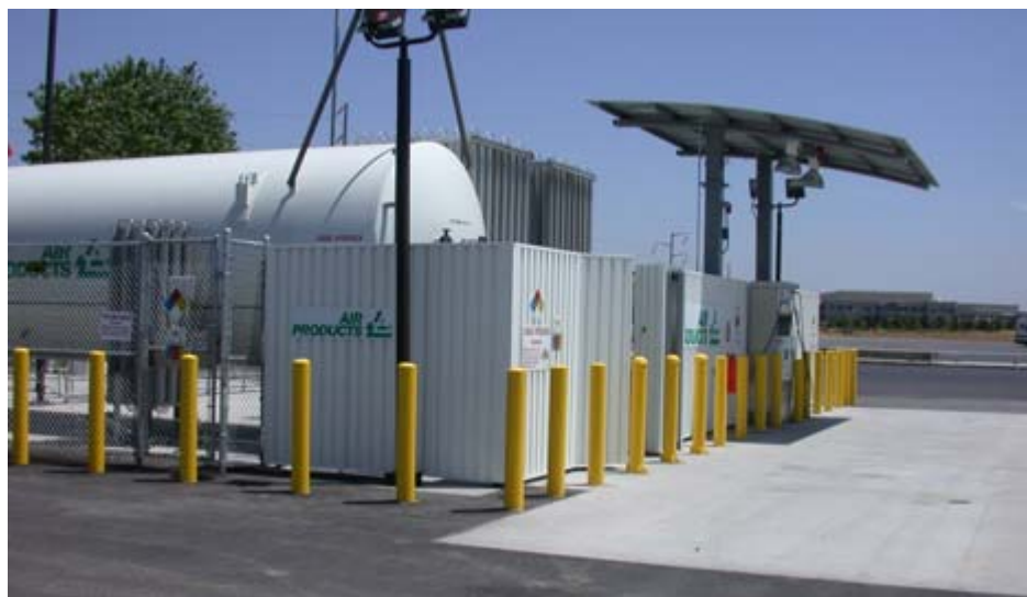
Figure 3. Compressed Hydrogen Dispensing Station at VTA's Cerone Operations Division
