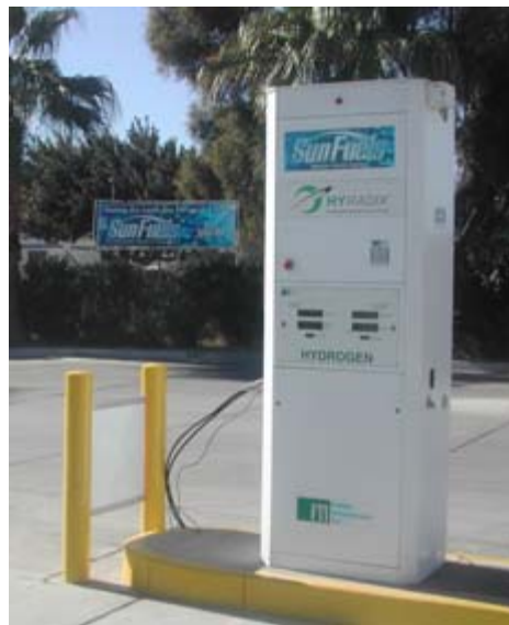
Figure 14. Hydrogen dispenser at SunLine
