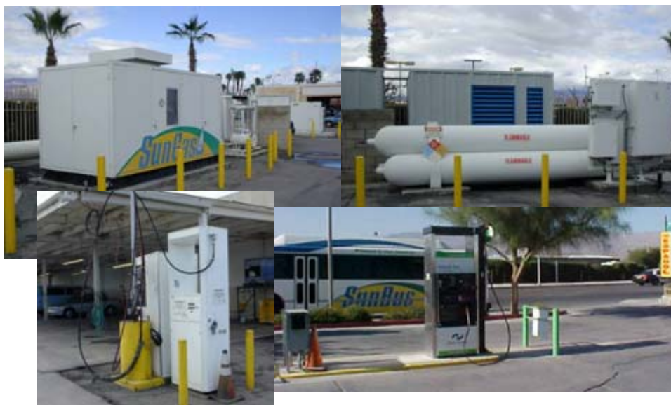
Figure 10. CNG fueling equipment (Indio)
