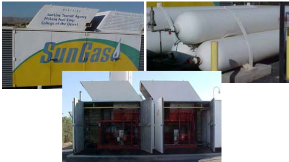
Figure 9. CNG compressor station (Thousand Palms)
