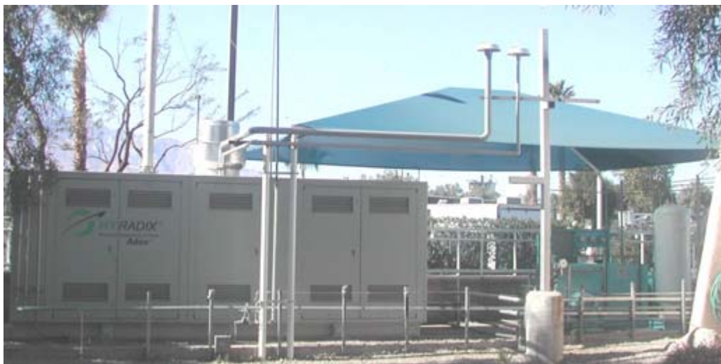
Figure 12. HyRadix natural gas reformer
