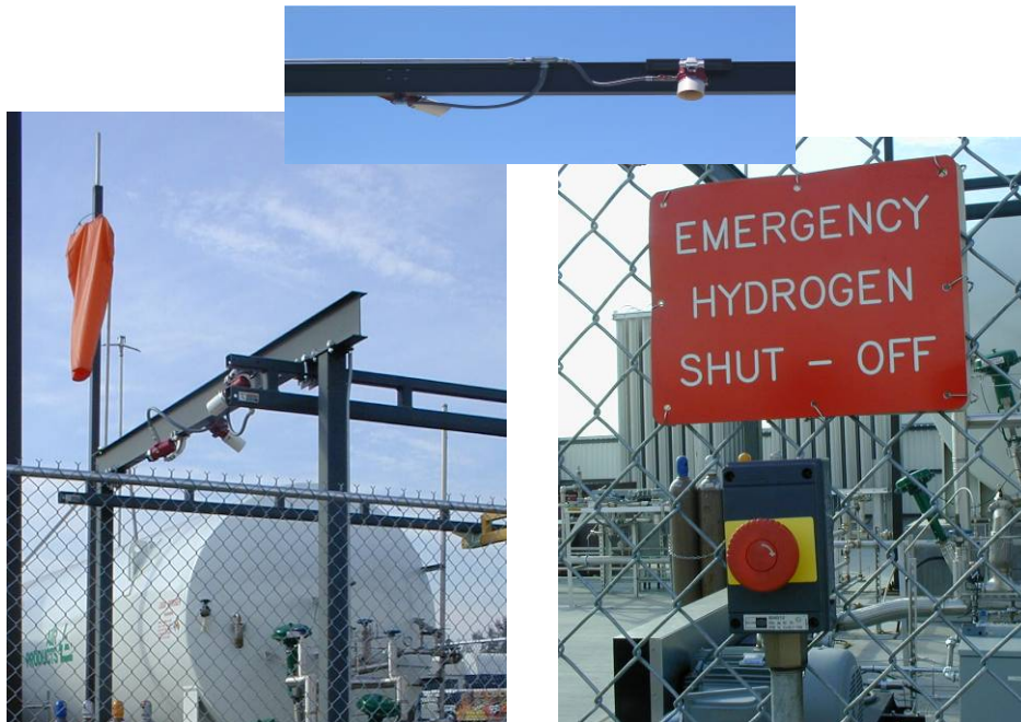
Figure 6. Flame sensors (left and top) and emergency shut-off (right) at the hydrogen dispensing facility
