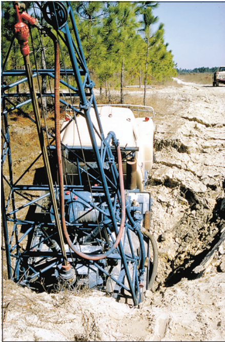
Figure 22. "A giant sink hole opened up on Thursday, September 19 [1975] at a drilling site near Tampa, Florida and swallowed up a well-drilling rig, a water truck, and a trailer loaded with pipe all valued at $100,000. The well being drilled was down 200 ft when the ground began to give way to what turned out to be a limestone cavern. Within 10 minutes all the equipment was buried way out of sight in a crater measuring 300 ft deep, and 300 ft wide. Fortunately, the drilling crew had time to scramble to safety and no one was hurt." -from National Water Well Association newsletter. (Photograph courtesy Tom Scott.)
