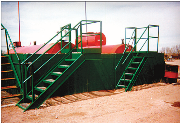
Figure 17b. Properly constructed containment facilities can protect the aquifer from potential fuel spills. (Photograph courtesy Lafarge.)
