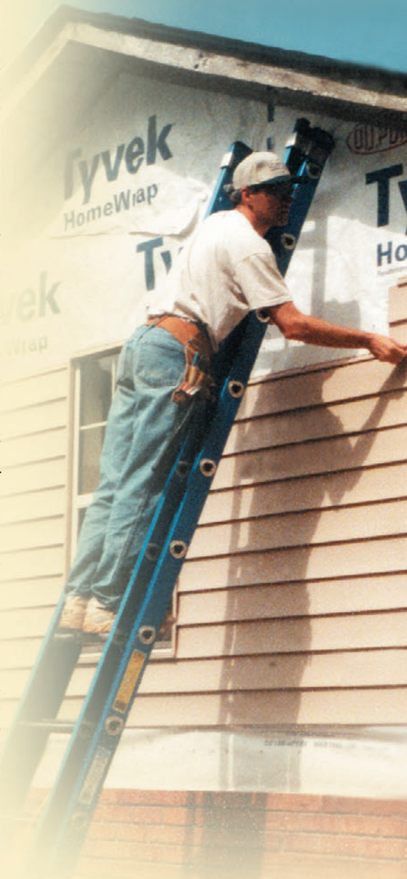
This Habitat for Humanity house being built near ORNL will produce as much energy as it uses, making it a zero energy building. ORNL was the first organization to use Habitat for Humanity houses to test energy-efficient building concepts.
