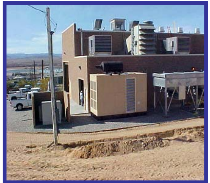
View of turbine hall with black-start generator outside building. CHP system is on line.
