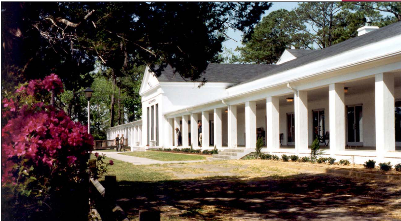
A GHP retrofit of Camp Lejeune's Marston Pavilion conference center is underway.
