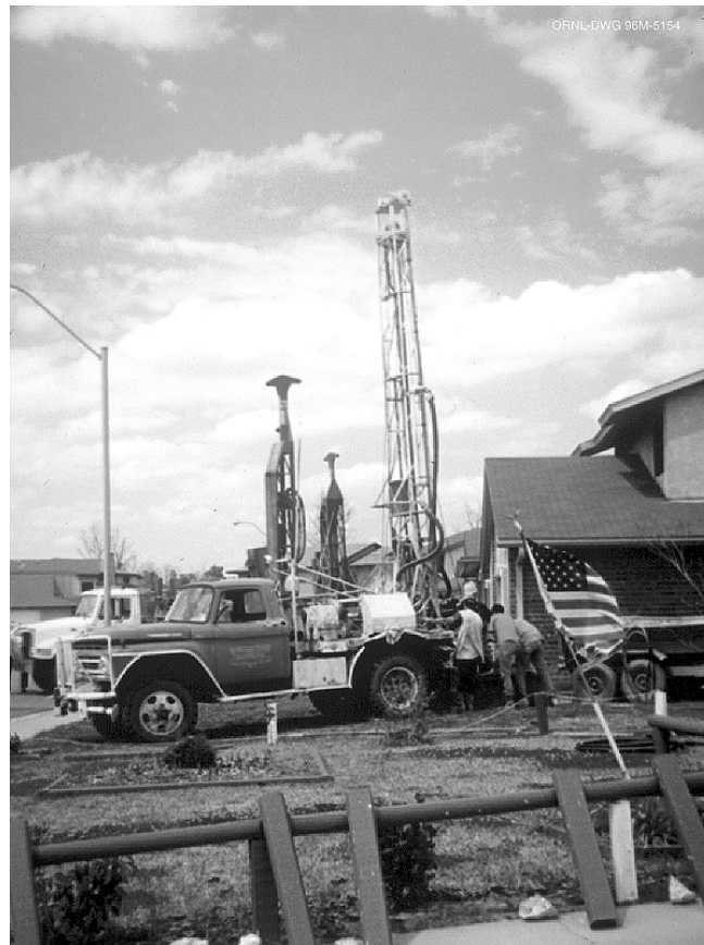
Fig. 1.4. A rig drilling vertical boreholes for the ground heat exchangers. A total of 1,834,652 ft of 4 1/8-in. vertical bore was drilled for the vertical borehole heat exchangers.
