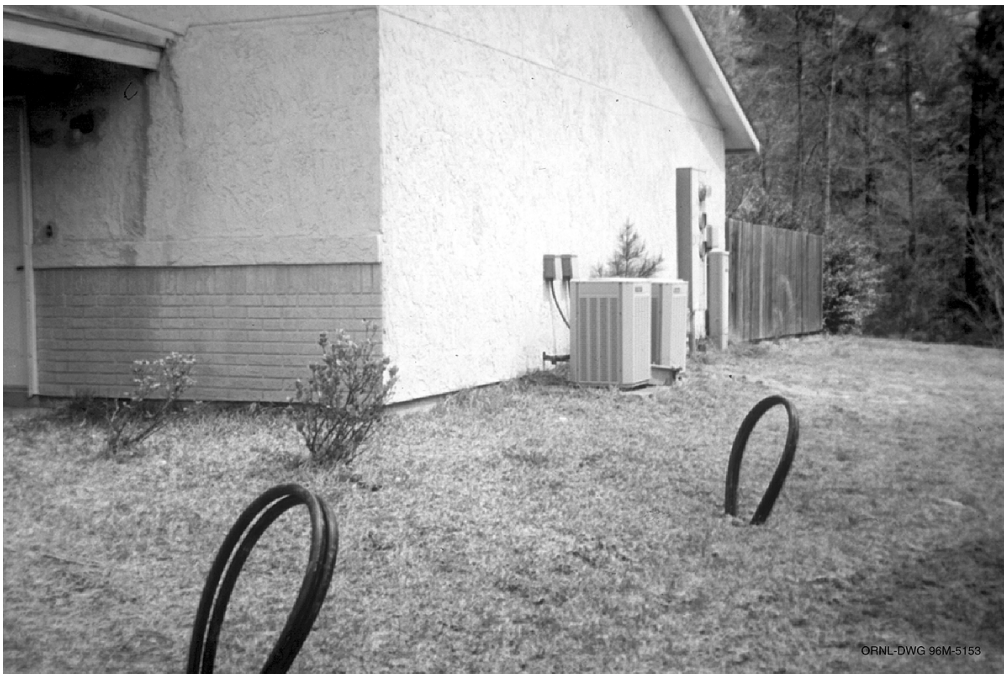
Fig. 1.6. Above-ground loops of pipe show where ground heat exchangers have been installed and are ready to be connected to heat pumps.
