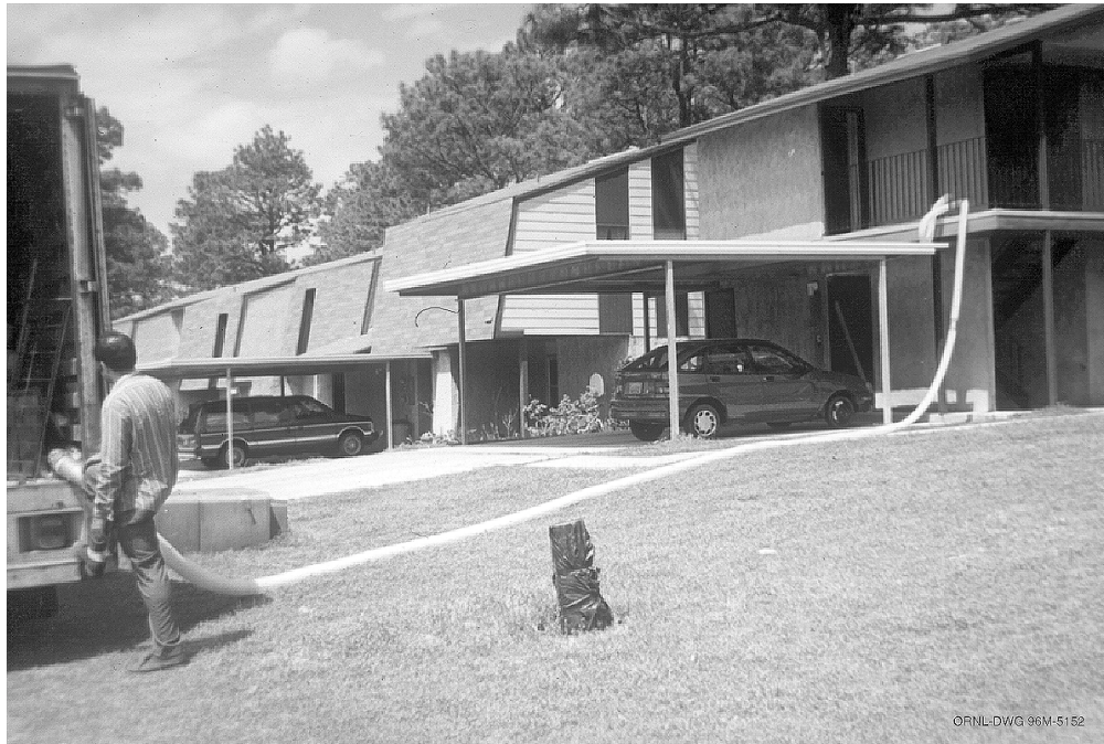
Fig. 1.2. Family housing apartment buildings at Fort Polk. Attic insulation was installed in some apartments as part of the energy retrofit.
