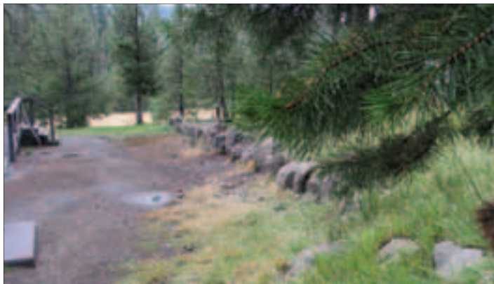
West of the lodge a single-course, dry-laid retaining wall separates the parking lot from the lawn area. Photo, 2003. (National Park Service)
