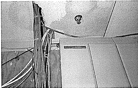
Photo 5 – State Office 6: Water sprinkler is leaking directly above the telephone, power, and computer lines.
