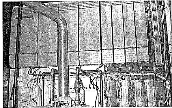
Photo 6 – State Office 2 Hot water tank and water supply lines are in front of the telephone and power lines.
