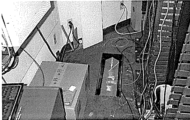
Photo 3 – State Office 6: Behind the server racks is again used for storage. Employees walk over server plugs and cables to get to storage items.
