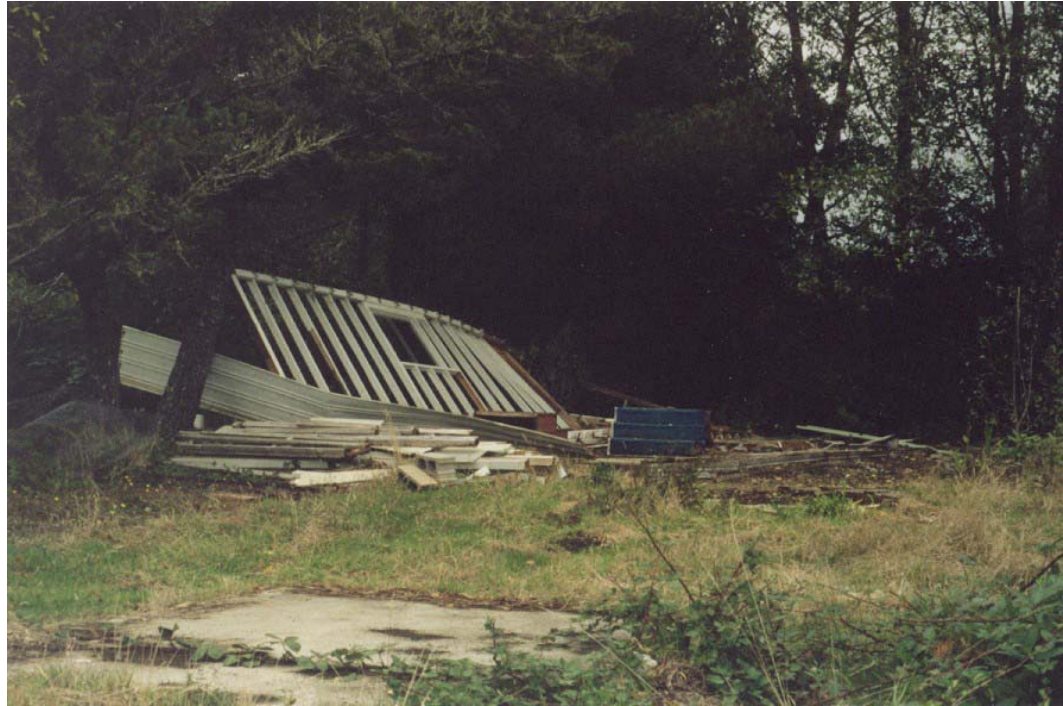
Figure 1: Deteriorating structure that the public could inappropriately access.(OIG Photo)
