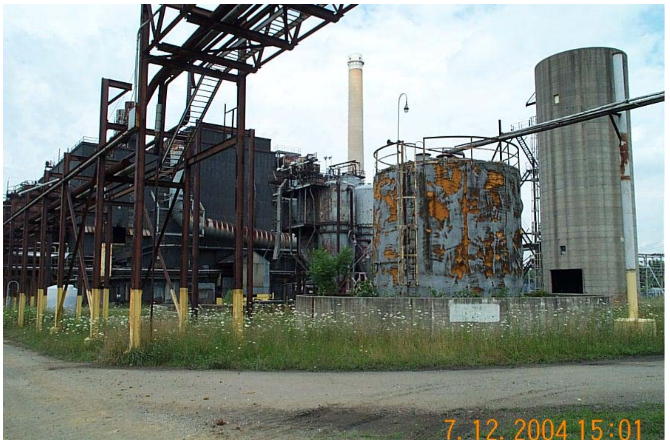
July 12, 2004, photograph of the inoperative boiler at the Biomass South Point, Ohio facility.
