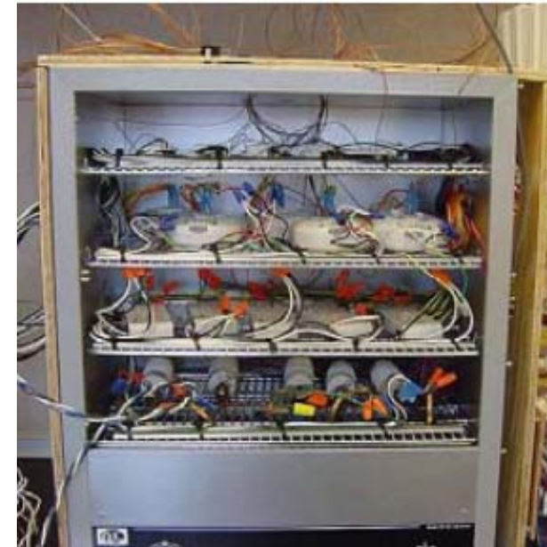
Ballasts and lamps inside thermal chamber used in ACTV test
