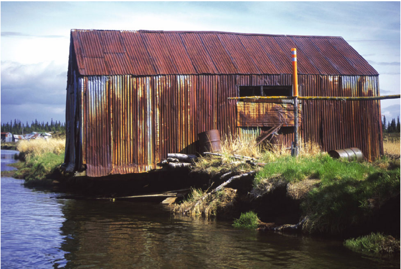
Figure 21. Bank erosion beneath bankside structure, Alagnak River river kilometer 17. Photograph by author, June 5, 2001.
