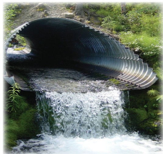
Rich Creek culvert before replacement. Kootenai National Forest
