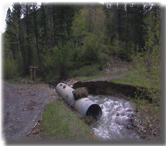
Washed out culvert, Helena National Forest
