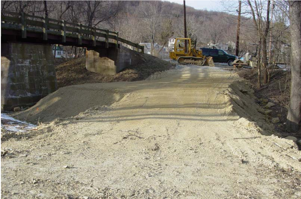
Construction of temporary causeway. Pivot bridge structure to left. White filter fabric visible in left center.
