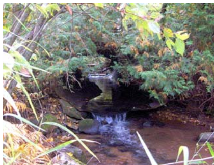
View of a perched culvert creating a fish barrier on Billy Creek in the Bad River Watershed. The old culvert was also failing structurally and erosion was occurring on both the downside and upstream side of culvert.
