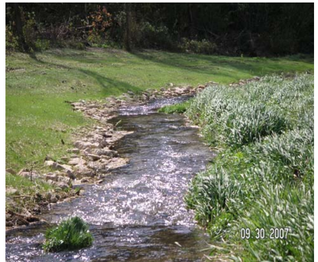
Post construction -Improved stream velocity. Weirs were installed to create pools. Boxelder was removed. Photo courtesy H.&L. Nohr Chapter TU.
