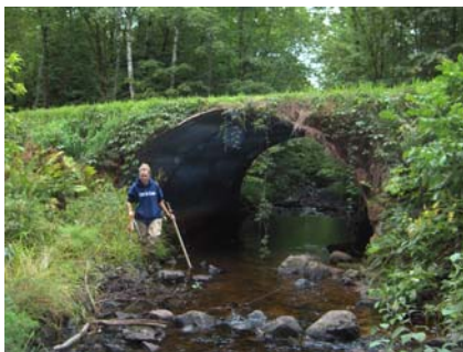
A culvert on Trout Brook in the Bad River Watershed. The inventory identified several fish passage and other problems: it is perched approximately 1.5 feet, the culvert bottom is rusting away, the cover over the culvert is less than 1 foot and it is not embedded. (photo taken looking downstream)
