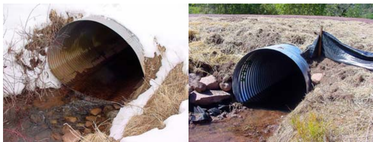
-USFWS photos A perched culvert (left) was replaced by a culvert which allows uninhibited fish passage on Little Whittlesey Creek that lies within the boundaries of the Whittlesey Creek National Wildlife Refuge.
