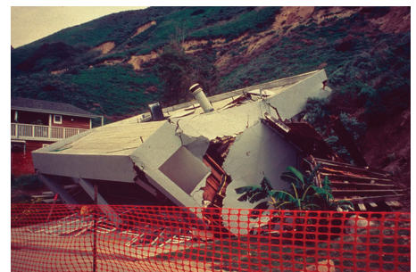
This house was crushed by the LaConchita, Calif., earth flow, Saturday, March 4, 1995. (USGS photo/Robert L. Schuster)
