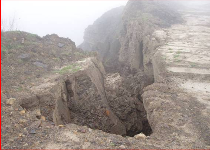
Figure 4. Block located 200 feet west of failure bounded by perpendicular joints has rotated from the highwall toward the pit, separating along a joint plane oriented parallel to the highwall. Block exhibits 12-foot separation with respect to the highwall.
