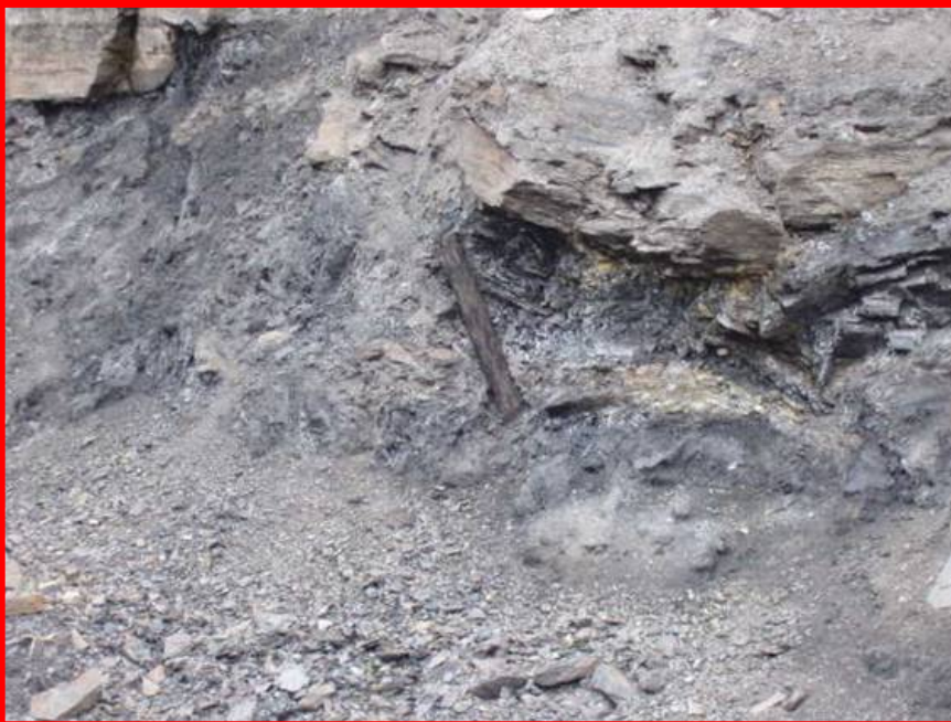
Figure 9. Wood post is preserved in crushed, in-filling rubble in a Pittsburgh seam room. Coal pillar is completely failed, characterized by extensive crushing and shearing, and illustrates the extent of damage in the Pittsburgh seam.
