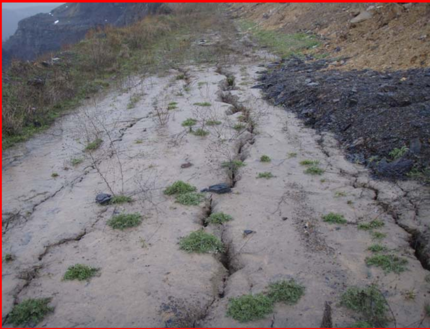
Figure 5. Rounded edges on middle tension crack indicate that it was present for a prolonged period, and most likely pre-dated the highwall failure. Swarm of cracks, present between the berm at the top of the highwall and the haul road, is oriented parallel to N 60-70° W-striking joint set. Area is located approximately 600 feet west of the failure.
