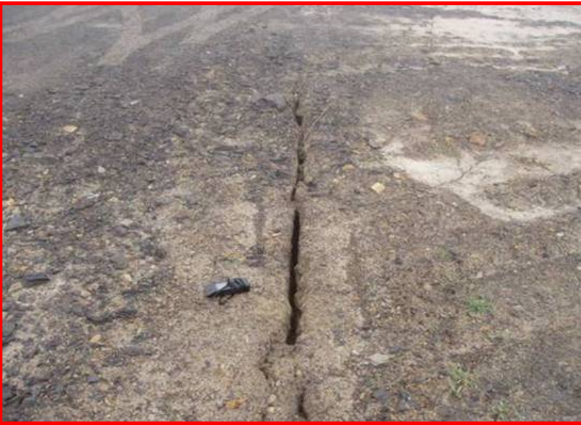
Figure 3. Open joint exposed at top of highwall, between the haul road and the highwall berm, exhibits aperture of three inches. Joint is parallel to trend of adjacent highwall.
