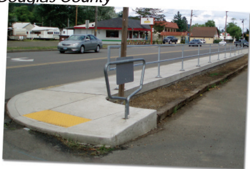
A project funded through ODOT's ESB program added sidewalk to the last unfinished segment along Central Avenue, Sutherlin's main thoroughfare.
