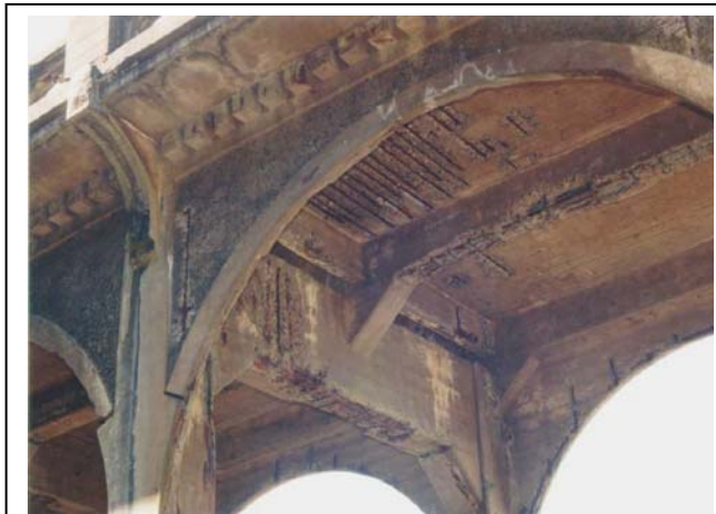
Structural deficiencies on the deck affect load capacity on the 76-year-old Old Winchester Bridge. (North Umpqua River in Douglas County)
