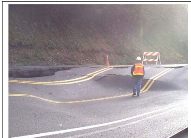
Salmon River Highway 18, on the way to the coast; 200 to 300 feet of damage;
