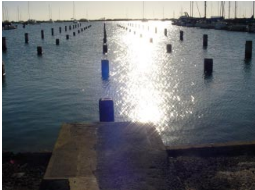
These pilings are all that remain from a collapsed pier at the Ke‘ehi Boat Harbor. Photograph courtesy of KMH LLP.
