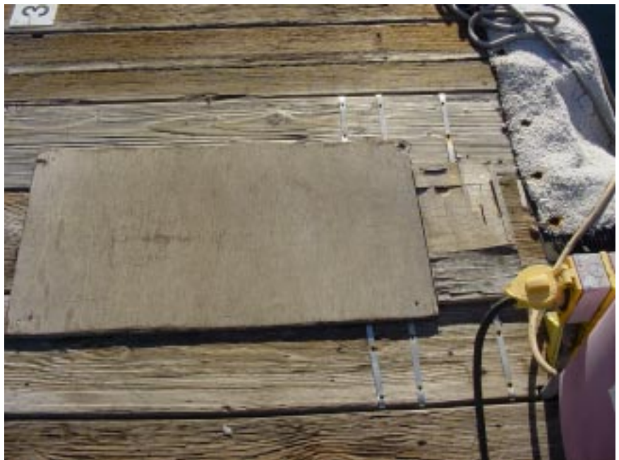
This Ke'ehi Boat Harbor pier has undergone numerous repairs after initial repairs failed. Photograph courtesy of KMH LLP.
