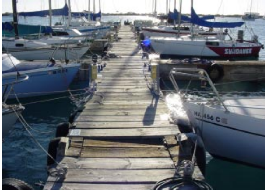
This Ke'ehi Boat Harbor pier poses a serious safety hazard. Photograph courtesy of KMH LLP.
