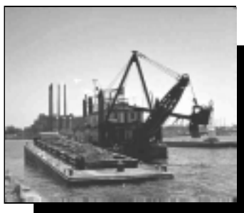
The dredging and safe disposal of contaminated sediments is a major step towards restoring the health of the Basin
