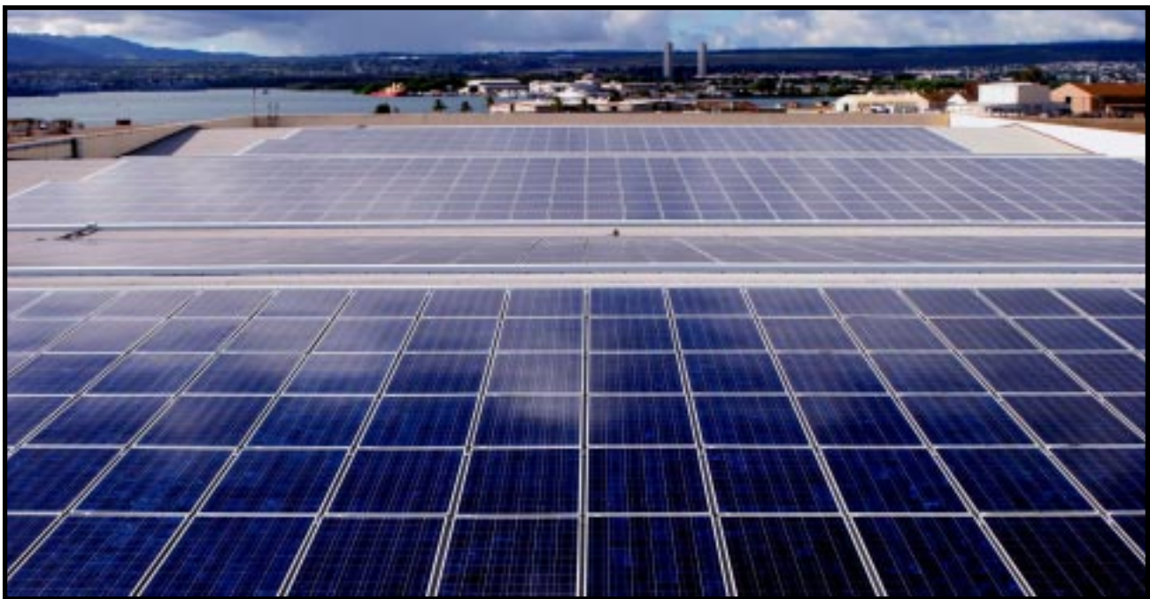
This Ford Island installation is Hawaii's largest federal solar electric system. Photo courtesy of PowerLight Corp.
