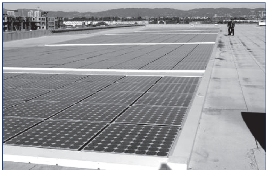
Figure 6. USPS Marina Processing & Distribution Center PV Array (G. Marsh, PIX 11015).
