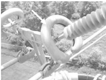
Energized End Grading Ring
