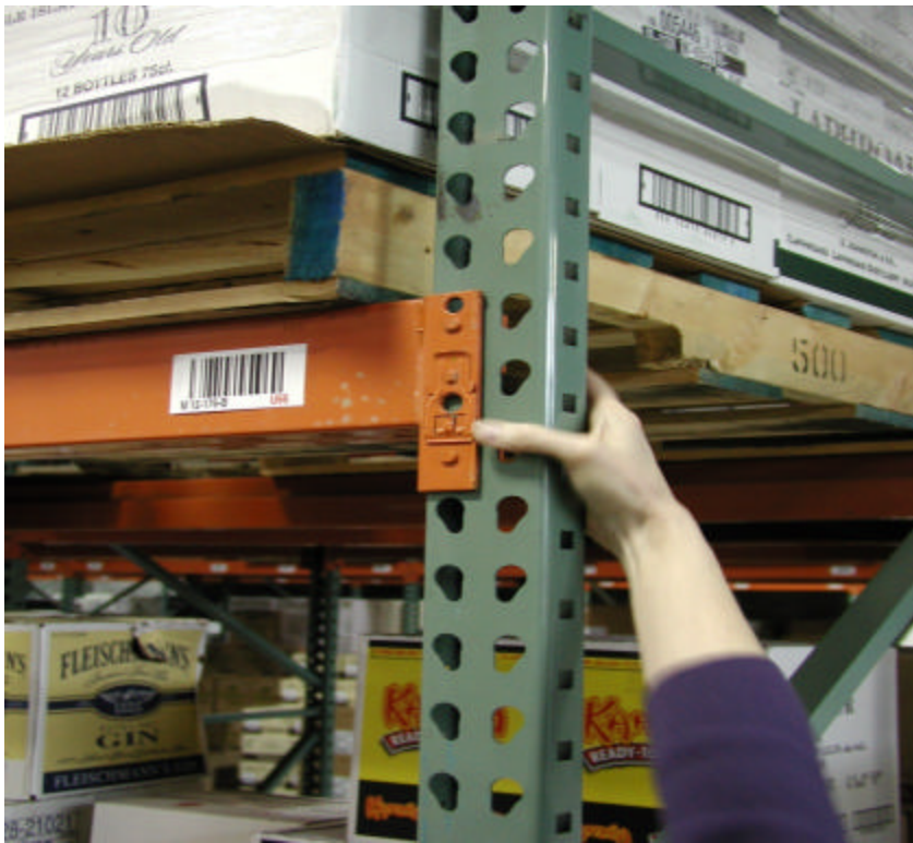
Figure 7. Spring clips on racks at the Oregon Liquor Control Commission warehouse.
