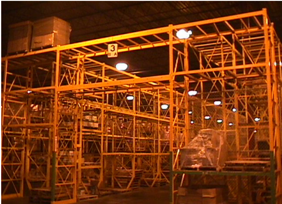
Figure 5. Racks on the main floor of the Department of Corrections warehouse connected by horizontal braces as well as bolted to the floor.
