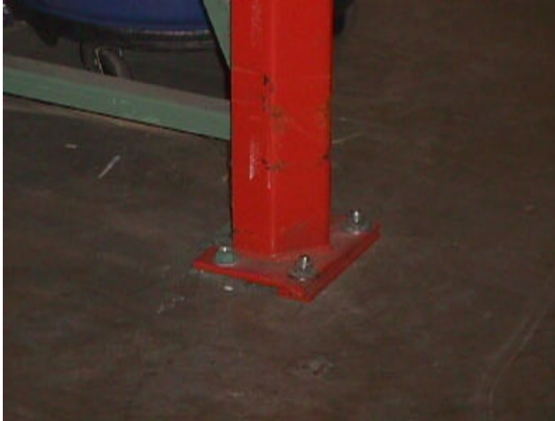
Figure 4. Racks bolted to the floor at the Oregon Lottery warehouse.
