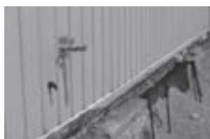
Coming from a bulk storage tank, this valve was left open and resulted in a 1,000 gallon spill. Notice the soil that was excavated due to contamination.
