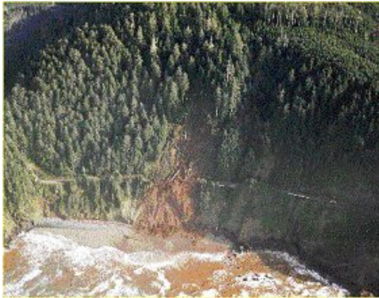
Figure 11. Cape Cove Landslide. A damaging landslide interrupted traffic in both directions of US Highway 101 in January 2000. Repair work forced an approximate three-month road closure. (ODOT photo)
