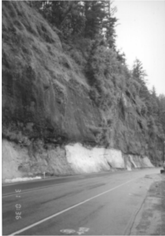
Figure 2. Various landslide control measures have been applied throughout the state. This photo shows the netting and shotcrete layer with drains on a road accessing the Columbia River Historic Highway, which experiences heavy traffic by tourists.
