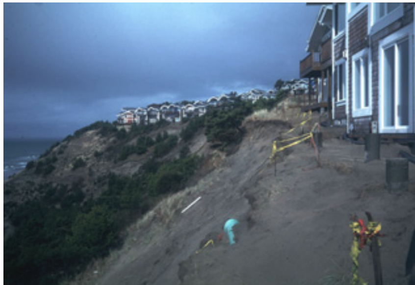
Figure 1. The Capes private housing community experienced landslide and coastal erosion damage associated with the 1997-8 El Nino event. Residents were evacuated and short-term mitigation was implemented. Long-term mitigation options, which need to accommodate coastal building regulations, are still being evaluated. Photo: Paul Komar
