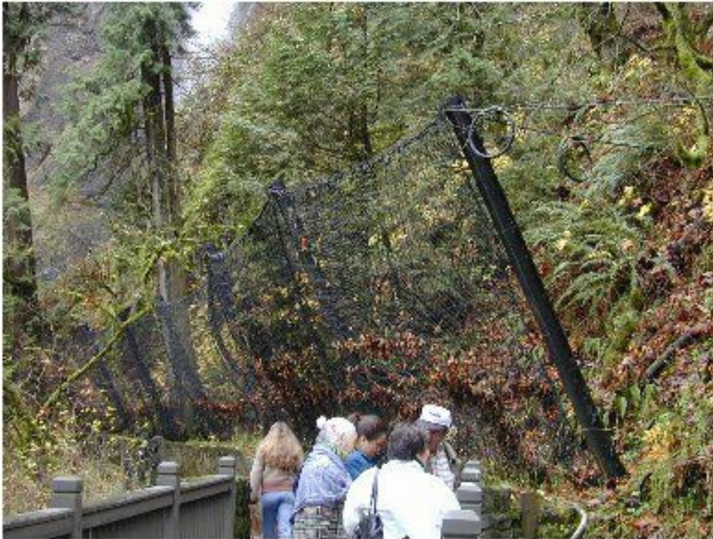
Figure 8. Multnomah Falls rock catchment net on footpath. This was installed by the USDA Forest Service as a result of a severe injury from a rockfall (modified from Wang and others, 2002)
