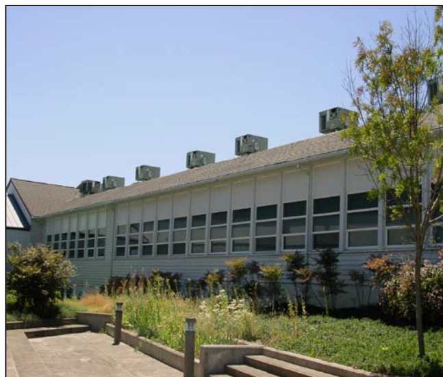
Philomath Elementary School has individual roof-top units for each classroom.
