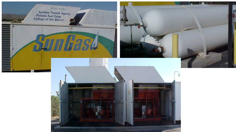
Figure C-3. CNG compressor station (Thousand Palms)
