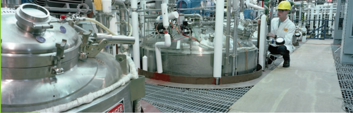
9,000-L fermentation tanks in the Biochemical Pilot Plant.
