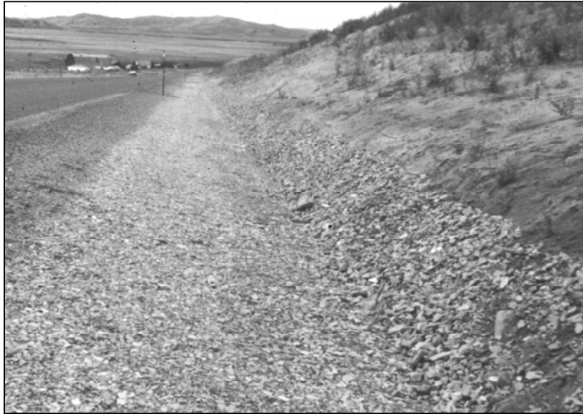
Figure 1.3. Cobble Channel Lining
