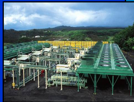
30 MW Puna Geothermal Power Plant, Hawaii
