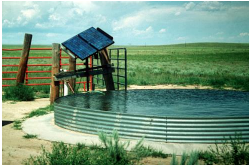
Solar Electric water pumping
