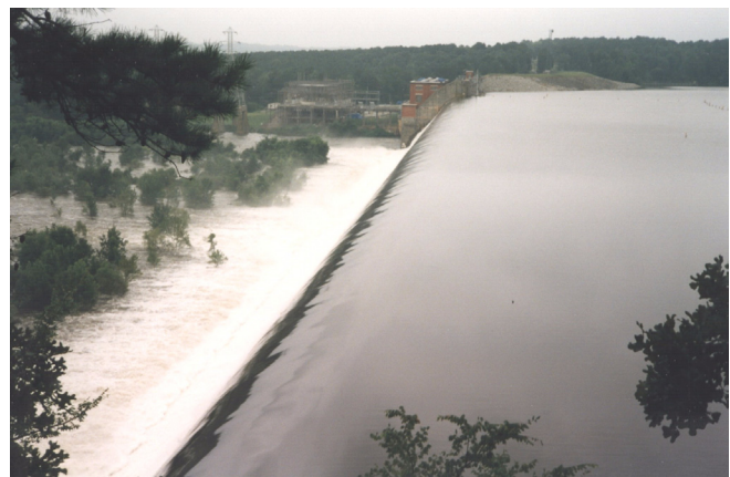
Wateree River dam being overtopped by high flows on July 25, 1997 (photo by Toby Feaster).
