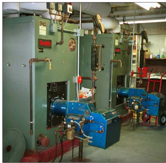
These boilers in the Warwick School District are operating very successfully with a B20 biodiesel blend. Photo: Bob Cerio
