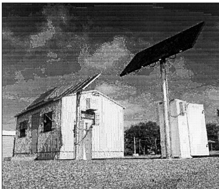
This stand-alone PV system consists of four modules, each with 36 cells. It provides power for lights, radios, televisions, and other loads at remote homes in New Mexico.
