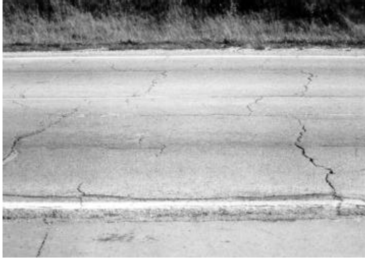
Figure 2. Pavement candidate for surface treatment: high-density cracking.
