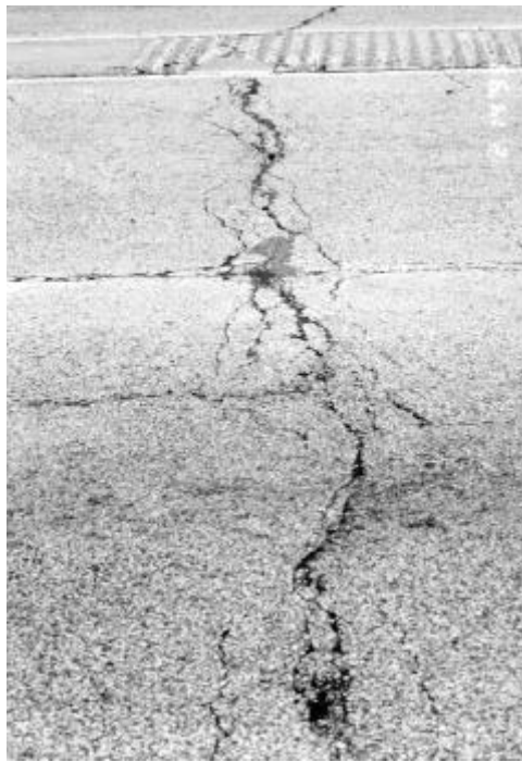
Figure 3. Pavement candidate for crack repair.
