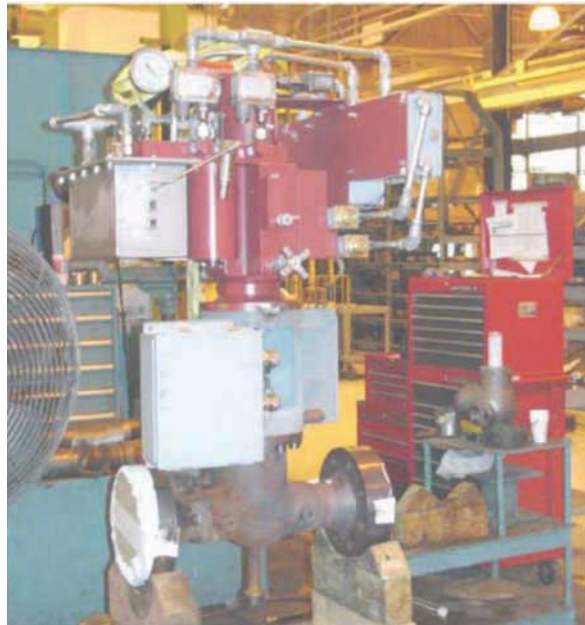
Figure 4 Size 4 Main Steam Isolation Bypass Valve
