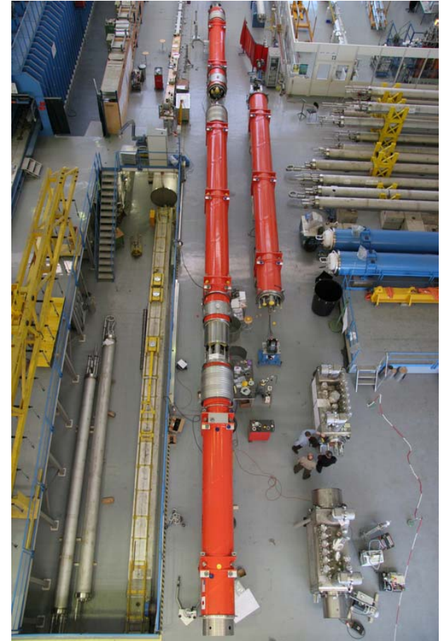
Q1 to Q3 aligned in 181. Q1 is at the bottom. Another Q2 and several BNL supplied dipoles are also visible
